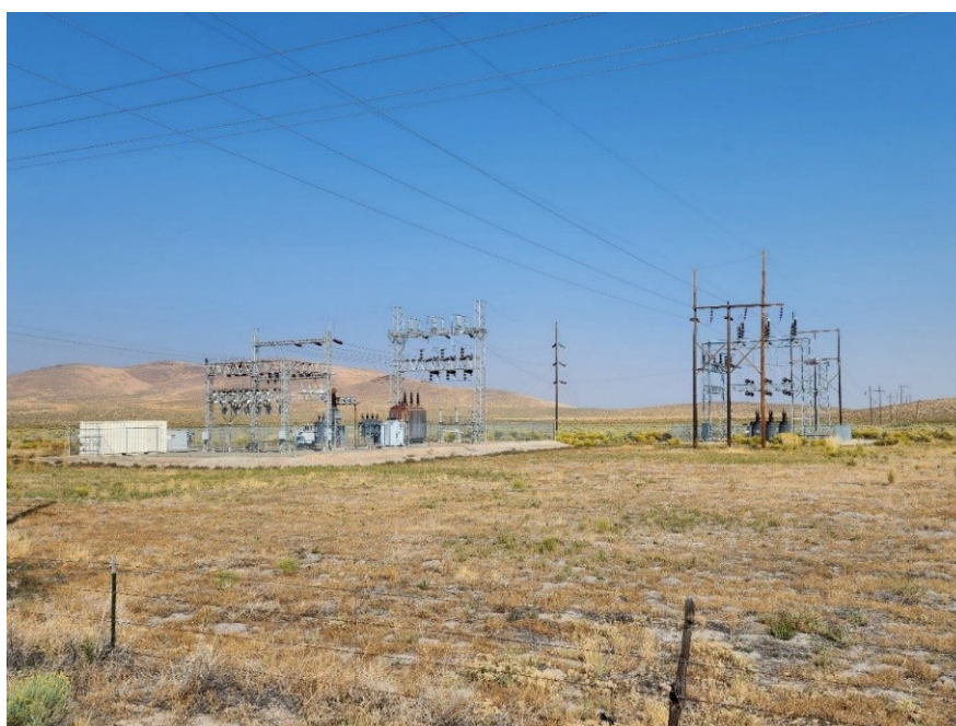
Figure 18. Existing HEC Substation located close to planned plant site.
