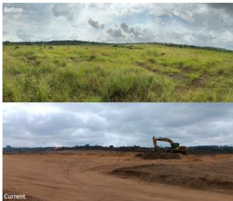
Figure 1 – Clearing work being completed at the Subantando Fertilizer Plant site, Cabinda, Angola.
