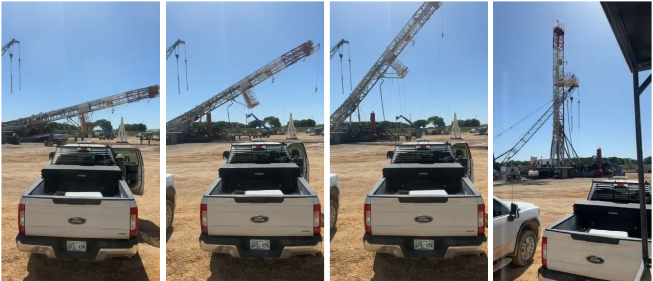
Figure 2: Raising of the Kenai Rig 19 derrick on the Rocket Well location, Flames Pad.
