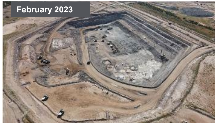
Stage 1 T3 open pit ~10M BCM mined, and pit progressed to ~60m depth
