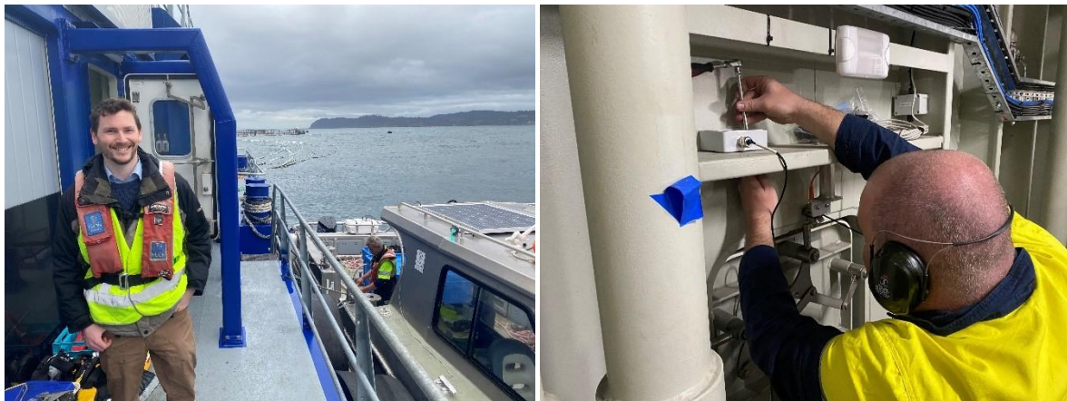
Instrumentation being fitted to operating aquaculture barge in Tasmania
