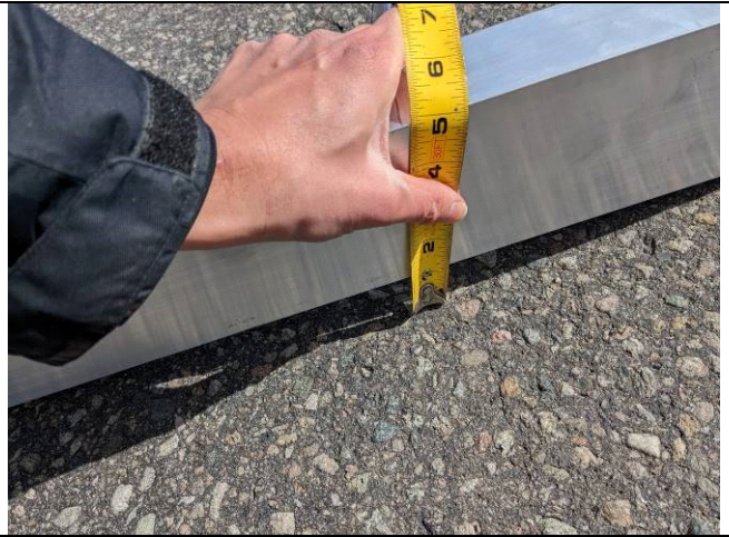
Asphalt Section 2, Rutting
