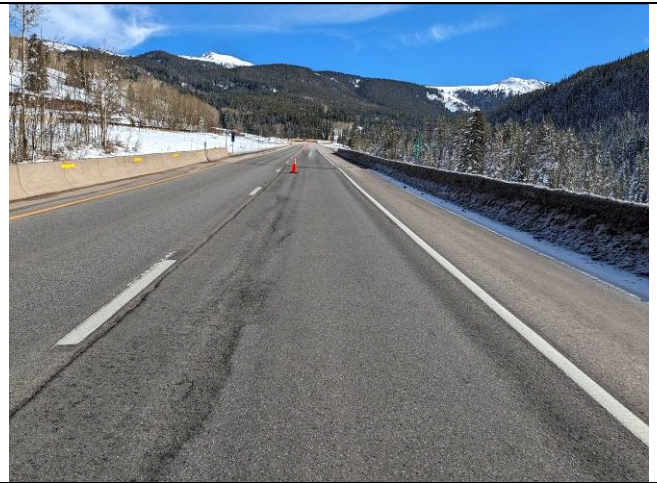
Rutting F-11-AM after Asphalt Test Section 1
