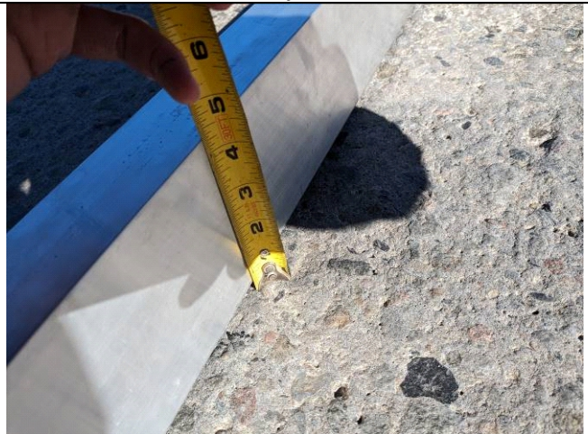
Concrete Test Section 1, Rutting
