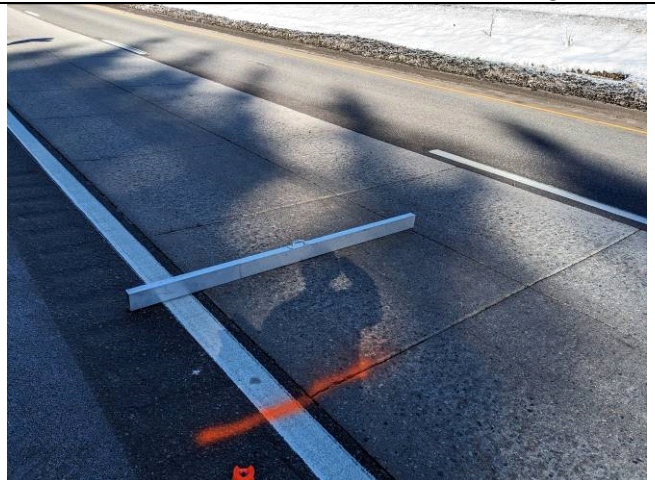
Concrete Test Section 2, Rutting
