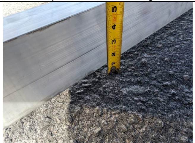
Asphalt Section 1, Rutting
