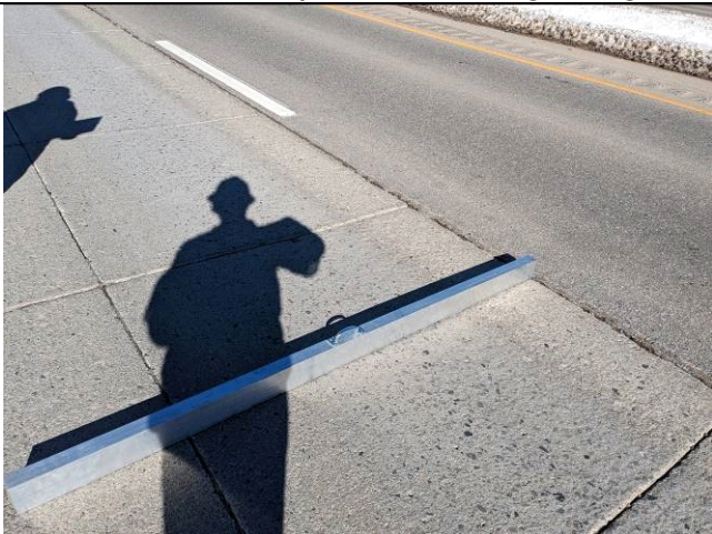
Concrete Test Section 1, Rutting
