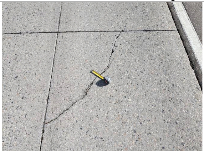
Concrete Test Section 3, Corner Break
