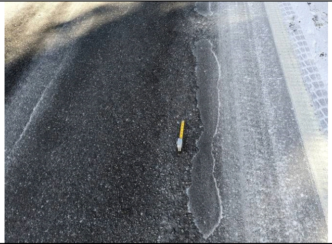
Asphalt Section 1, Rutting
