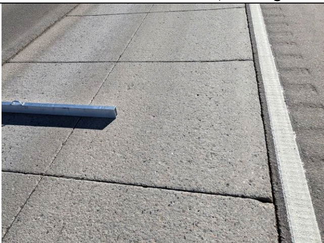
Concrete Test Section 1, Wheel Path and Minor Joint Spalling
