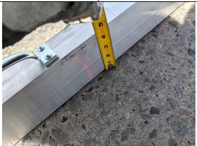
Concrete Test Section 3, Rutting
