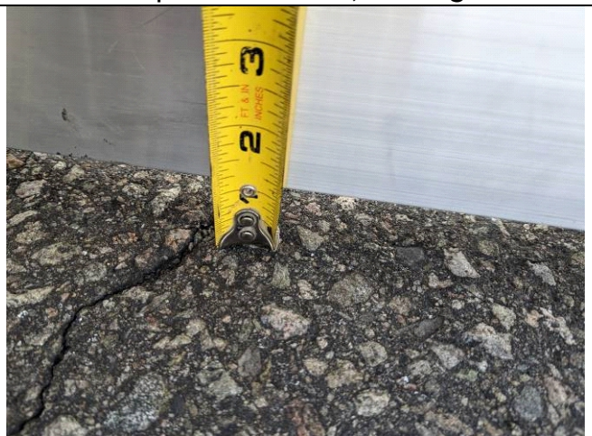
Asphalt Section 2, Rutting
