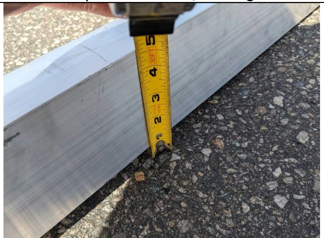
Asphalt Section 2, Rutting
