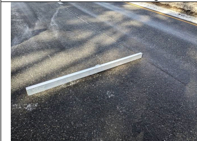
Asphalt Section 1, Rutting
