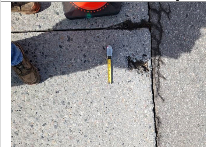
Concrete Test Section 3, Defect
