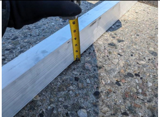
Concrete Test Section 2, Rutting
