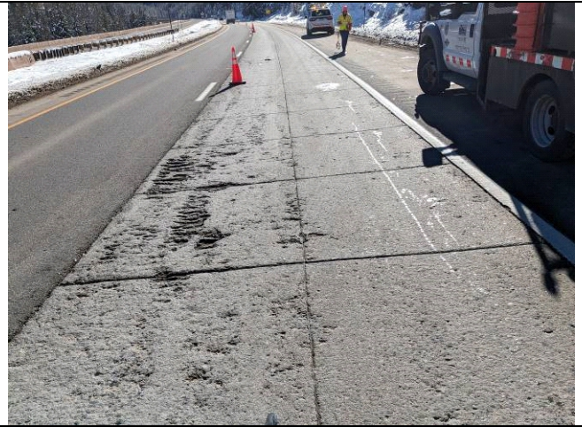
Concrete Test Section 1, Voids First 100 Feet
