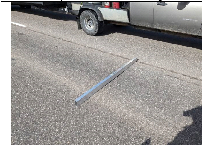
Asphalt Section 2, Rutting
