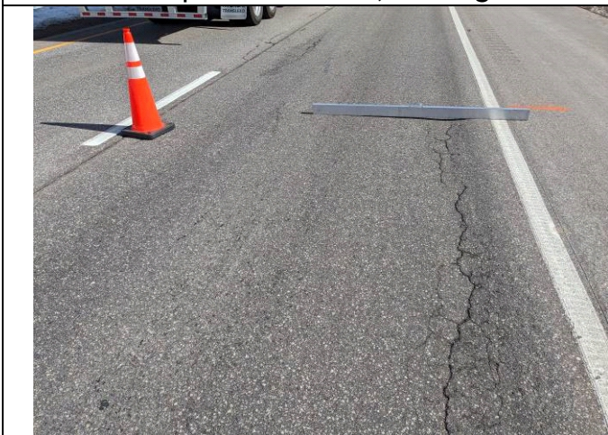
Asphalt Section 2, Rutting
