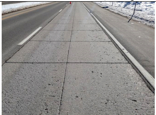
Between Concrete Sample Areas 1 and 2, Popouts
