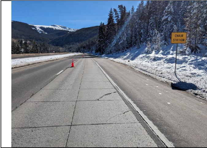
Between Concrete Sample Areas 1 and 2, Corner Breaks
