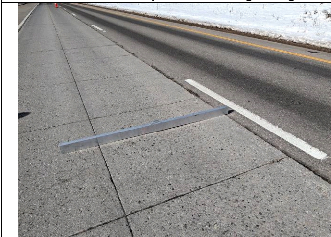
Concrete Test Section 3, Rutting
