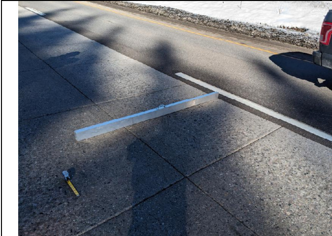
Concrete Test Section 2, Rutting
