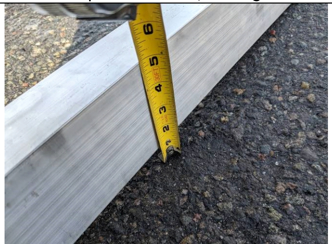
Asphalt Section 1, Rutting
