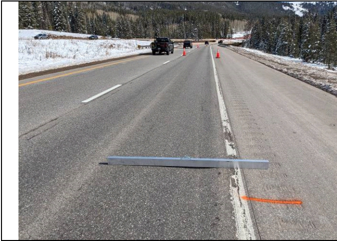
Asphalt Section 2, Rutting
