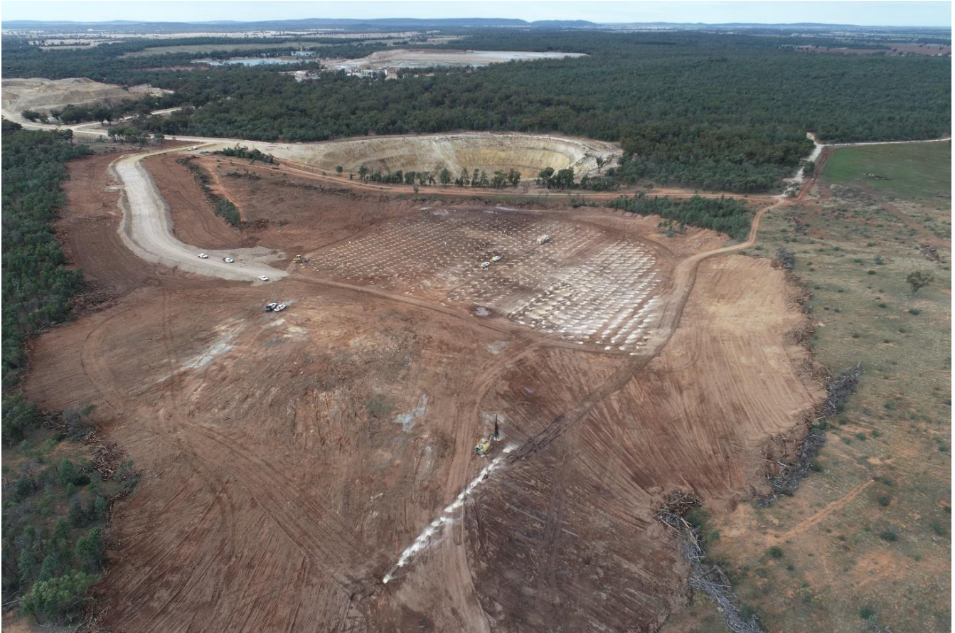
Figure 1: Pearse North – surface cleared, and first pattern drilled out, Pearse South open pit shown in the background. Mining initially commences in Pearse North and a cut back will commence on Pearse South.
