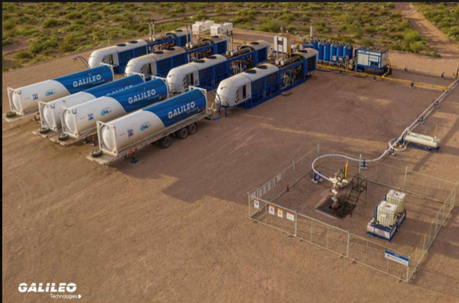
Drilling of additional production holes at existing Amersfoort field cluster followed by installation of micro-LNG train
