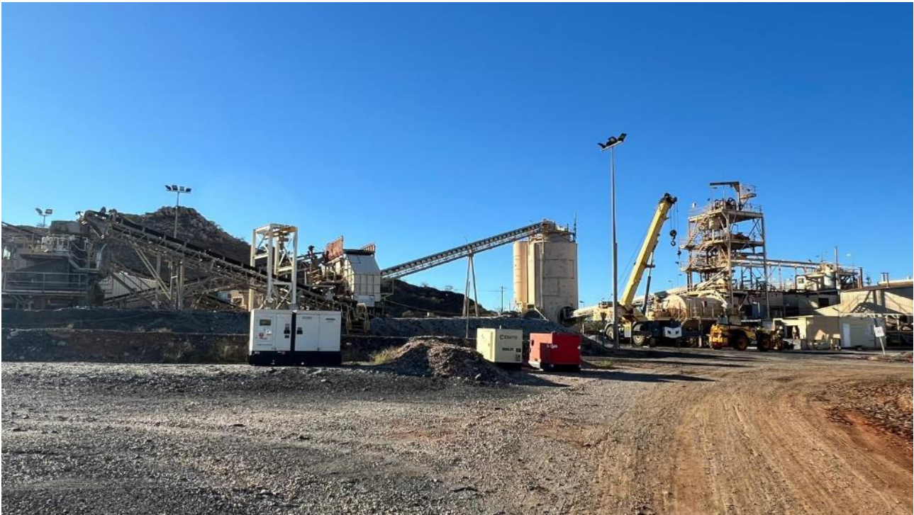
Figure 6: MACA equipment at the processing facility
