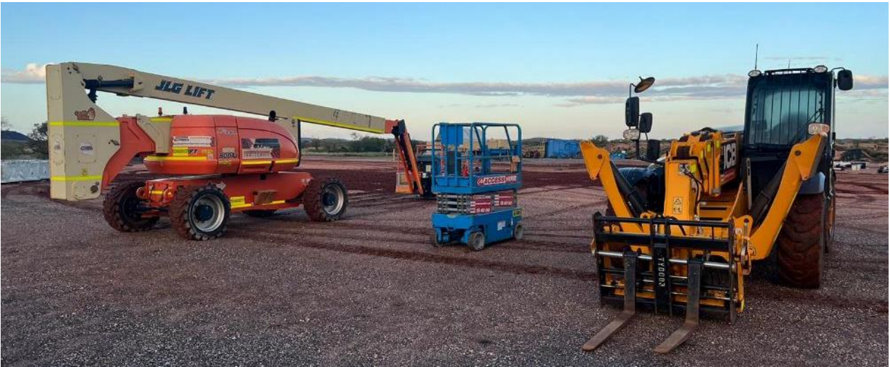
Figure 4: Newly delivered MACA equipment at the laydown yard
