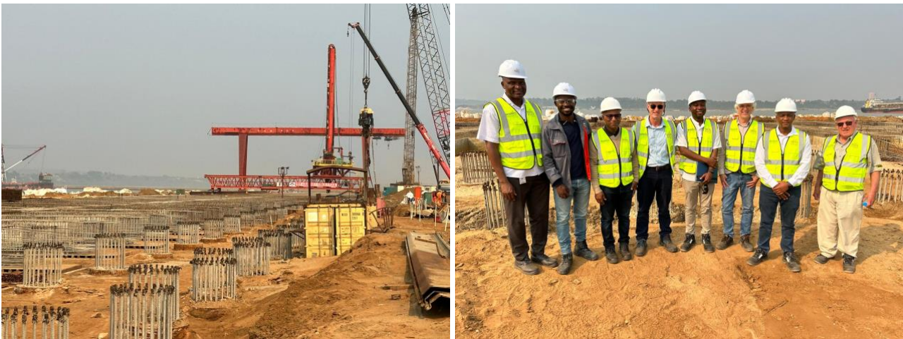
Figure 1. Visiting Porto do Caio Stage 1 Quay which is scheduled for completion in December 2025.
