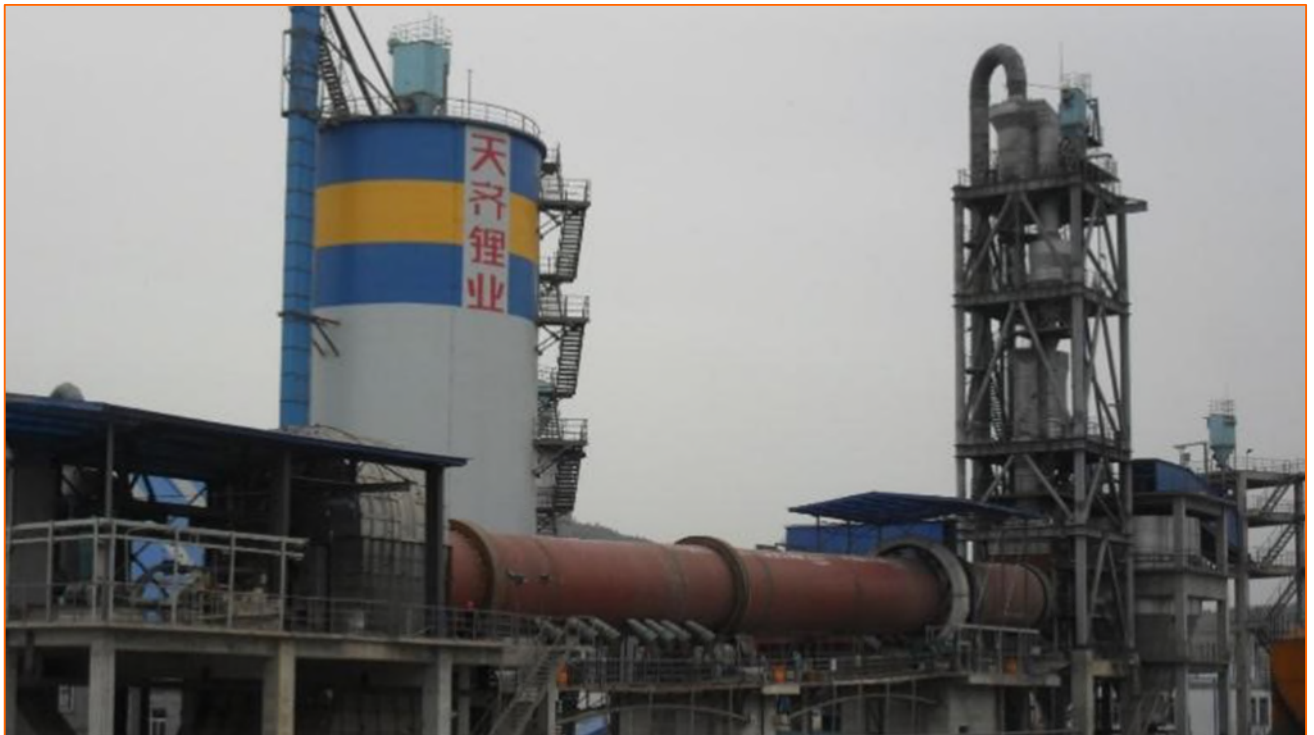
Figure 4: Typical natural-gas fired calcination kiln used in the lithium refinery process. Source: Sichuan Calciner Technology Pty Ltd
