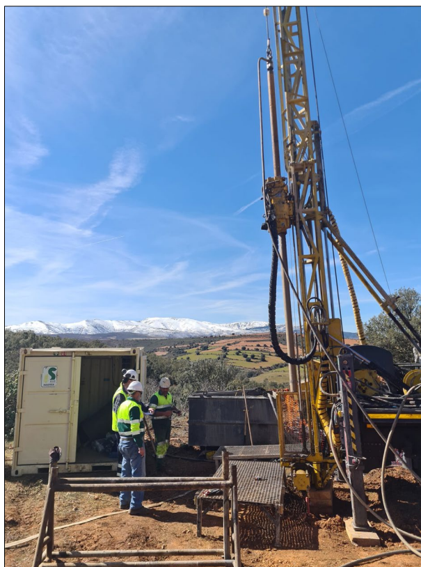
Figures 3: Drill rig commencing drilling at the Iberian One Project, Spain March 2024.
