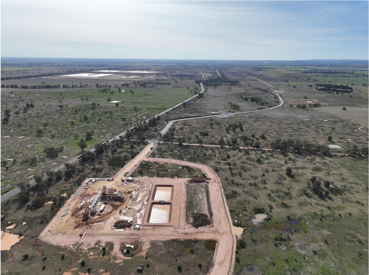
Internal light vehicle and pipeline corridor construction between Caloma Two and Roswell
