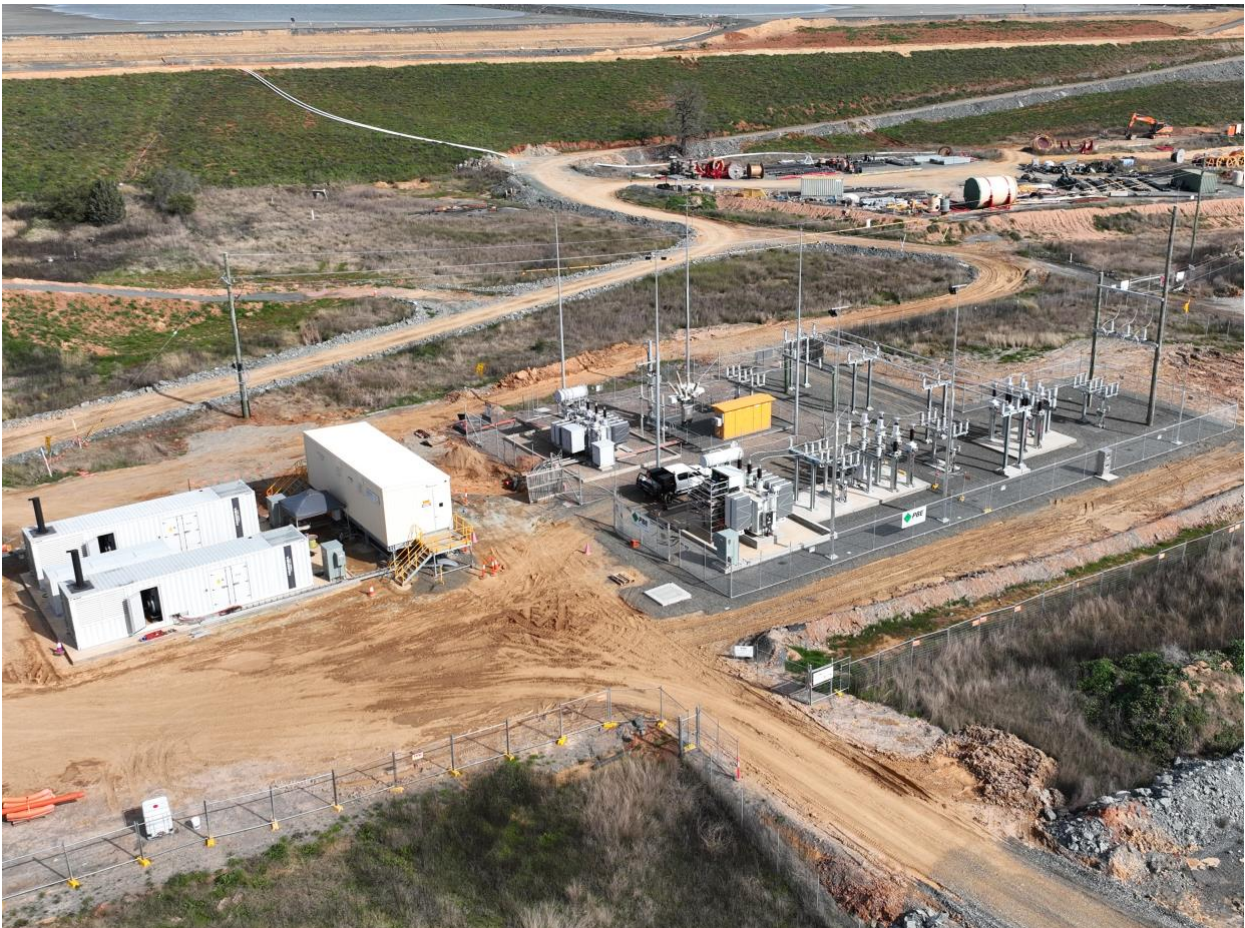
New 66kV yard (bottom yard) and generators
