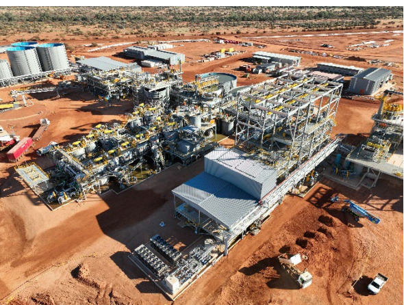
Figure 17: Aerial view of tantalum circuit
