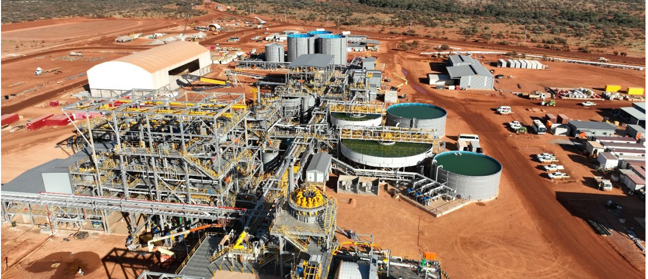
Figure 19: Aerial view of the Process Plant
