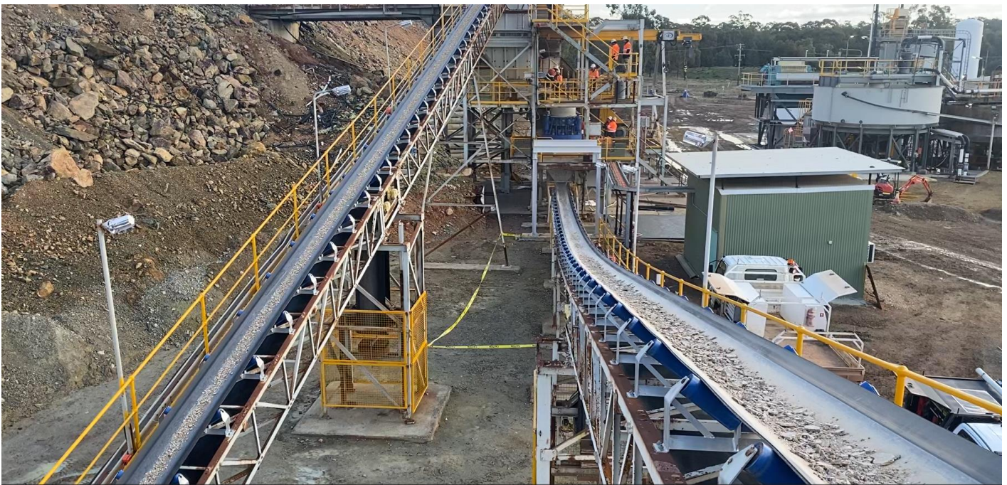
Figure 2: Pearse ore from the primary crusher on Conveyor 1 (CV1) & oversize returns on CV2 to the secondary crusher.
