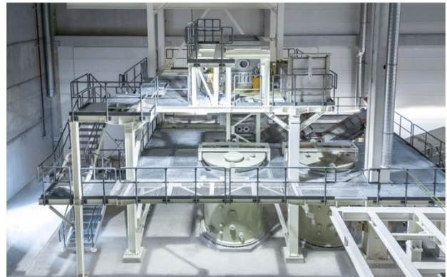
Figure 5 – Part of the Integrated LiB Plant installed by Primobius.
