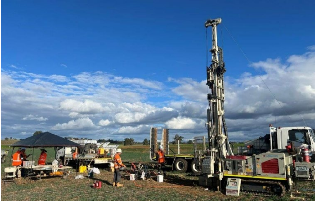
The Macquarie Geotech team has commenced work on the Dubbo Project site.
