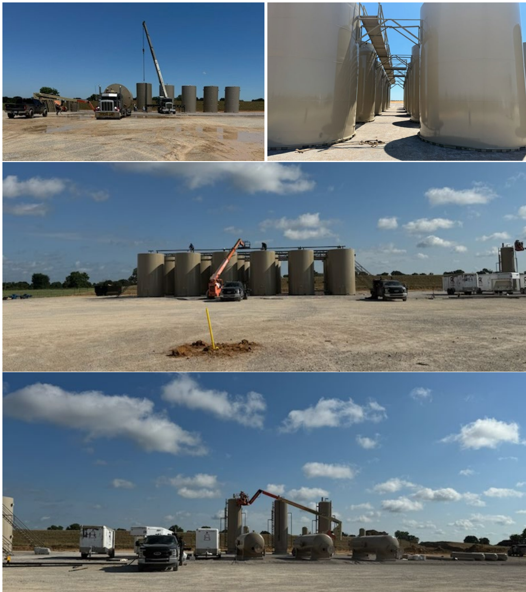
Figure 5: Setting of surface production equipment including the 18-tank battery on the Sanford Pad location.
