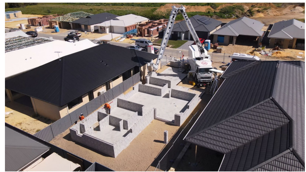
Hadrian X® building a structure in Perth, generating zero on-site masonry waste
