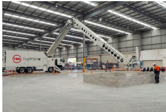
'Person in zone' (PIZ) operator inspects blocks that have just been laid
