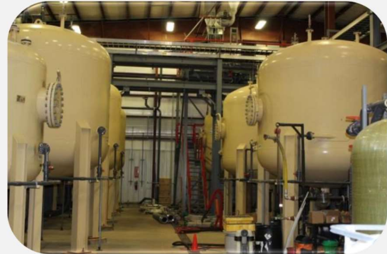
Satellite Plant Ion Exchange System
