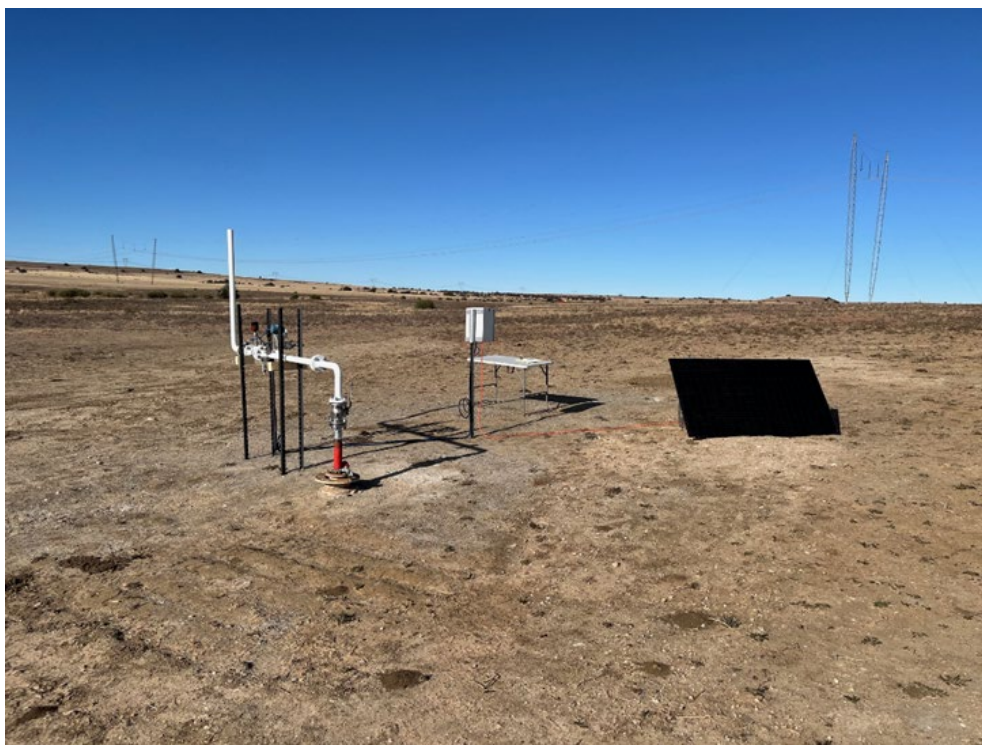
New Testing Equipment at RBD10
