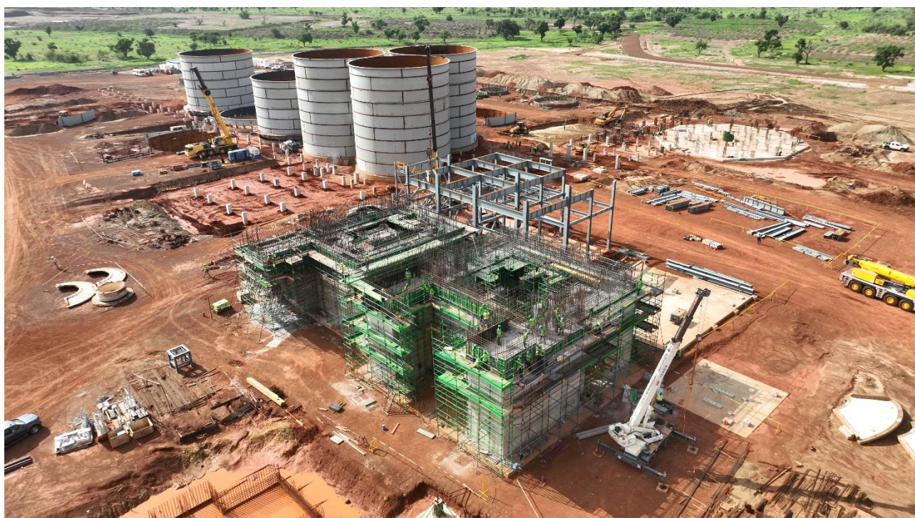
Construction of ball and SAG mill foundations, CIL tanks, and steel works at Kiaka
