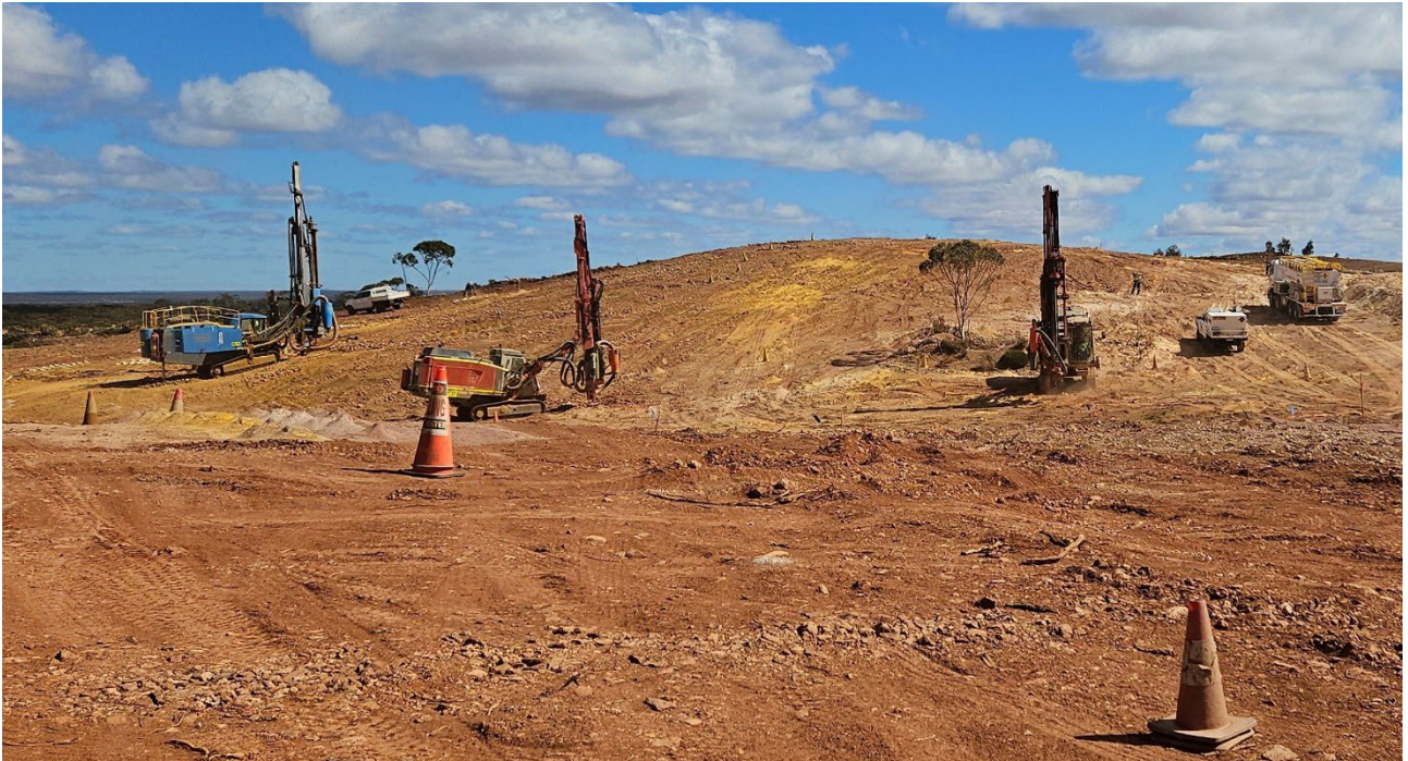
Figure 2: Grade Control (blue rig), blast hole drilling and loading first shot (23 August 2024)
