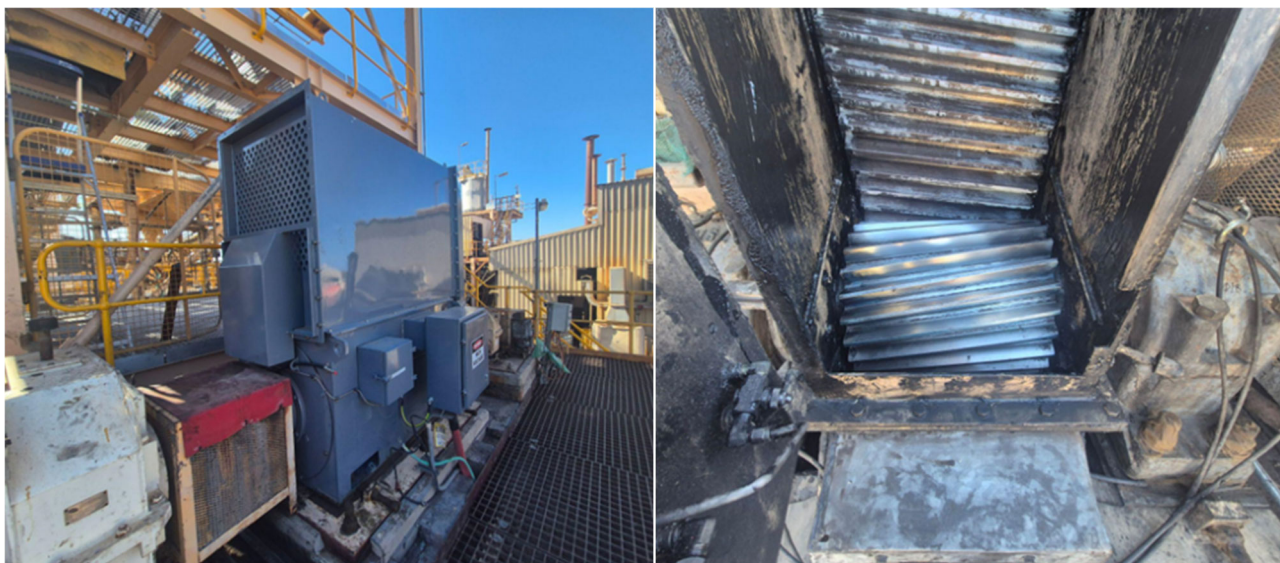
Figure 3: The refurbished ball mill motor has been installed and pinion gear installed and fully aligned.
