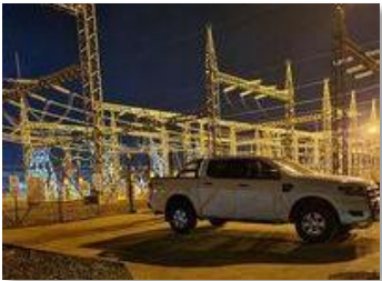
Eskom Substation 12km away
