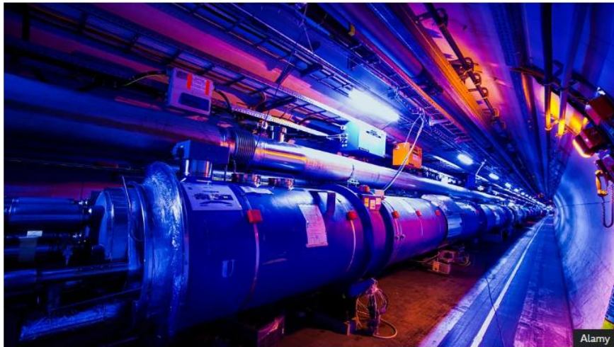
Liquid helium is used to cool the superconducting magnets at facilities such as the Large Hadron Collider (Credit: Alamy)
