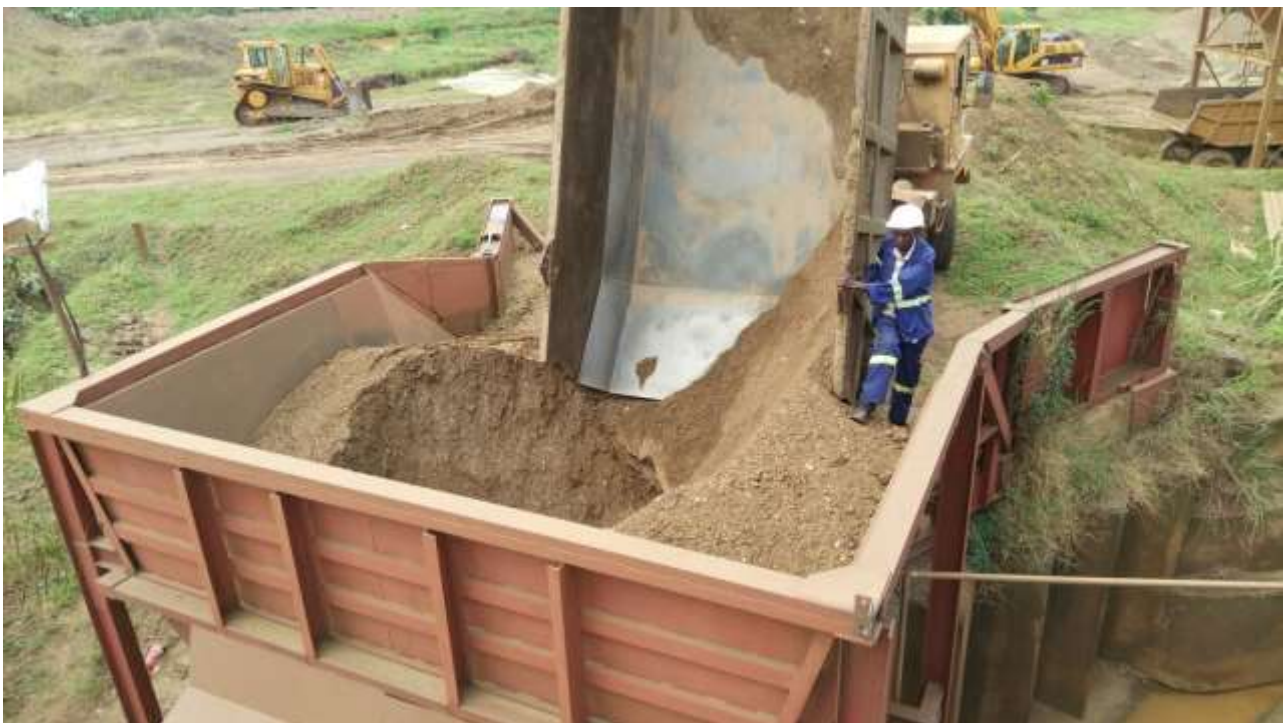
Vermiculite from the open pit mine tipped directly into the Run of Mine Bin - November 2016
