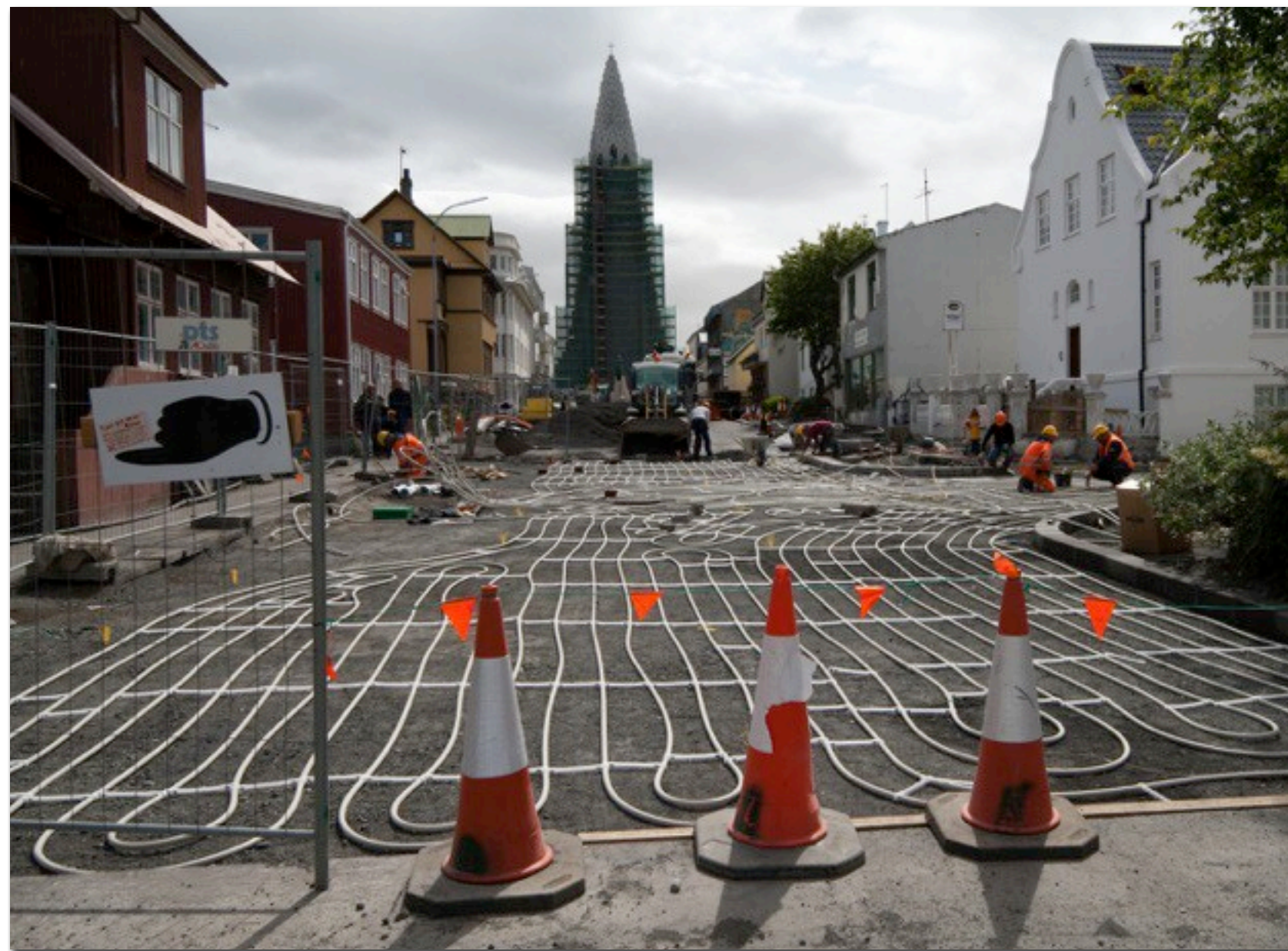
Snow & ice-free road heating installation
