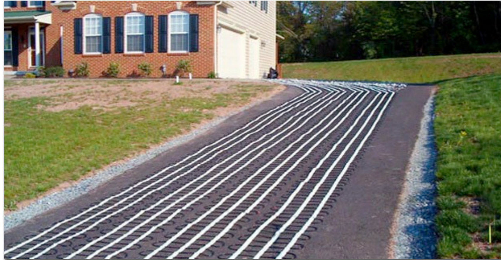
Snow-free driveway heating installation
