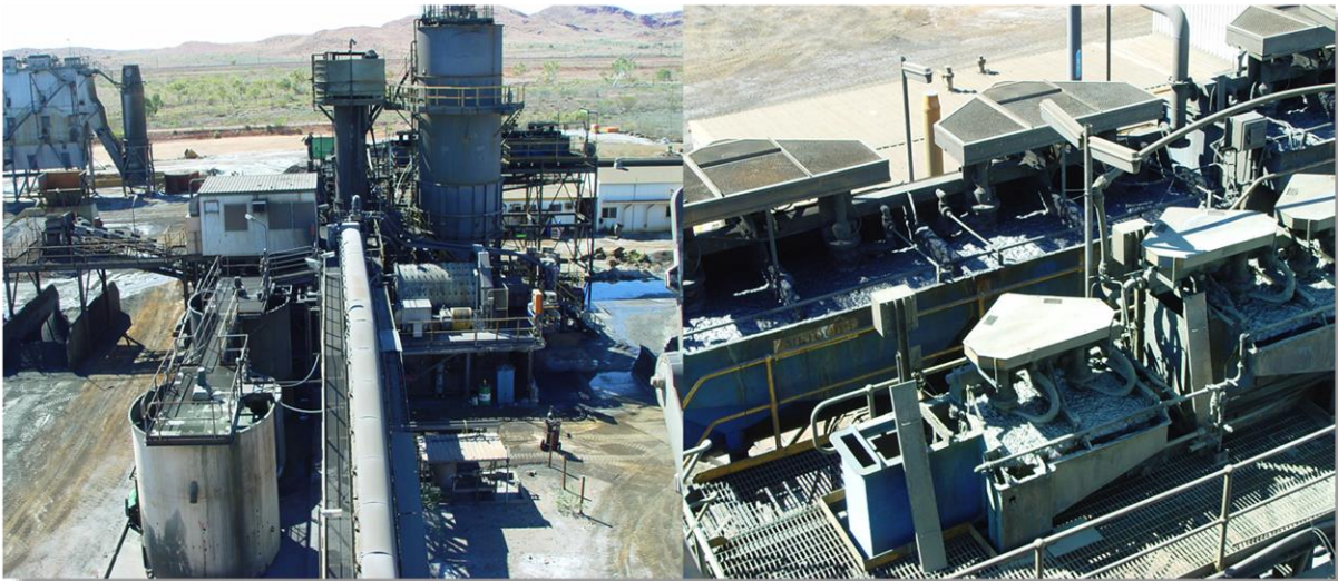
Figure 2a: AGIP Radio Hill Nickel/Copper Operations (Fox 100%) – Radio Hill 425,000 tpa Treatment Plant and flotation circuits.
