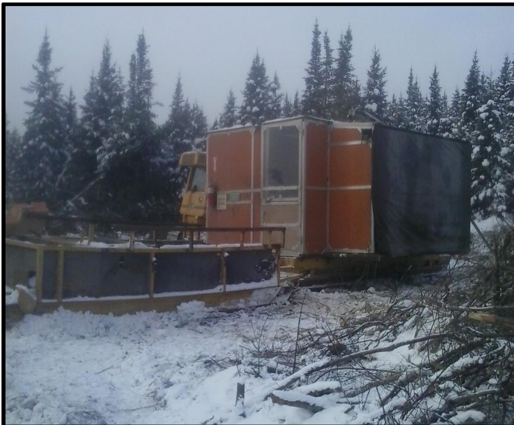
Figure 1. Diamond drill on site at the Manitouwadge Graphite project in Ontario, Canada.
