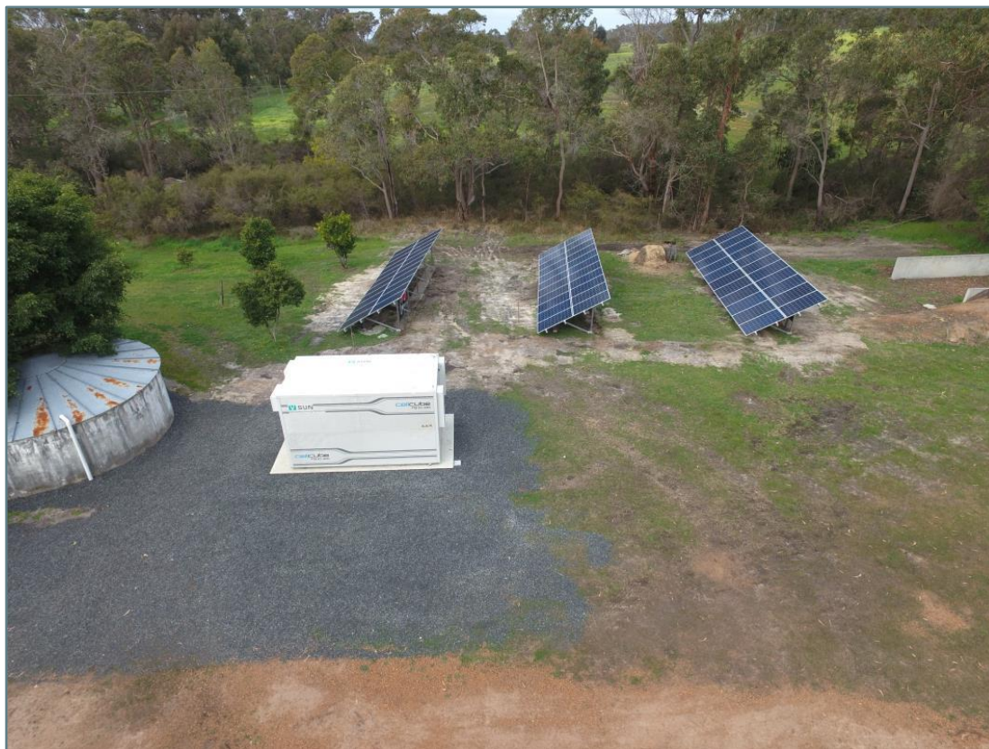
Plate 4. Busselton FB10-100 Installation and 15Kw PV System
