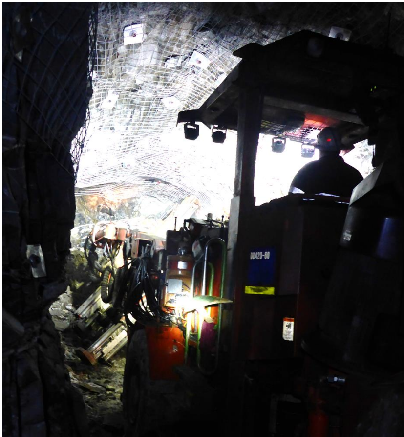
Figure 5. Mechanised (Jumbo) Development of the 1394 Ore Access Drive at the A1 Mine.
