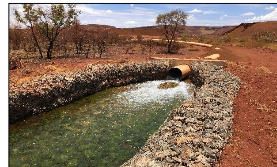
Iron Valley Dewatering Facility
