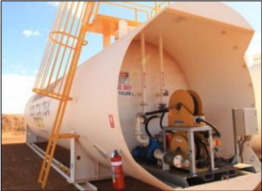
Figure 6-3: Self-bunded diesel tank
