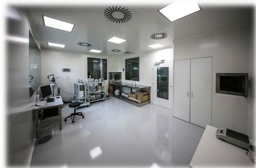
MXC's CO 2 Extraction unit in the European Clean Room Facility
