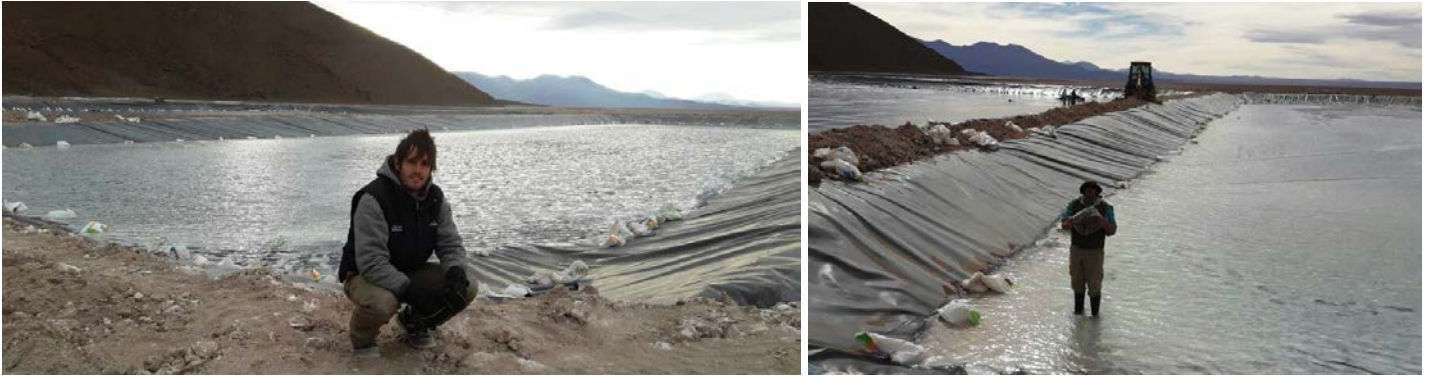
Photos 4 - 5. Rincon Lithium Project – First brine in ponds.
