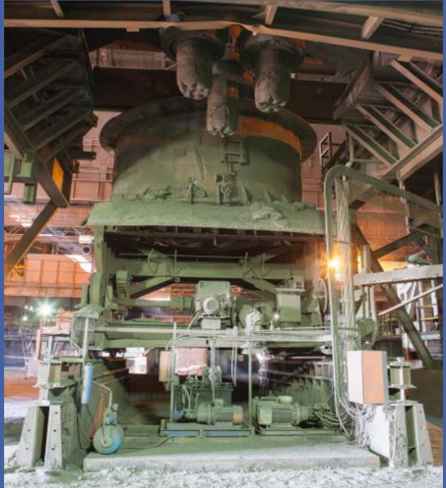
One of the two smelters in situ at Transalloys in South Africa
