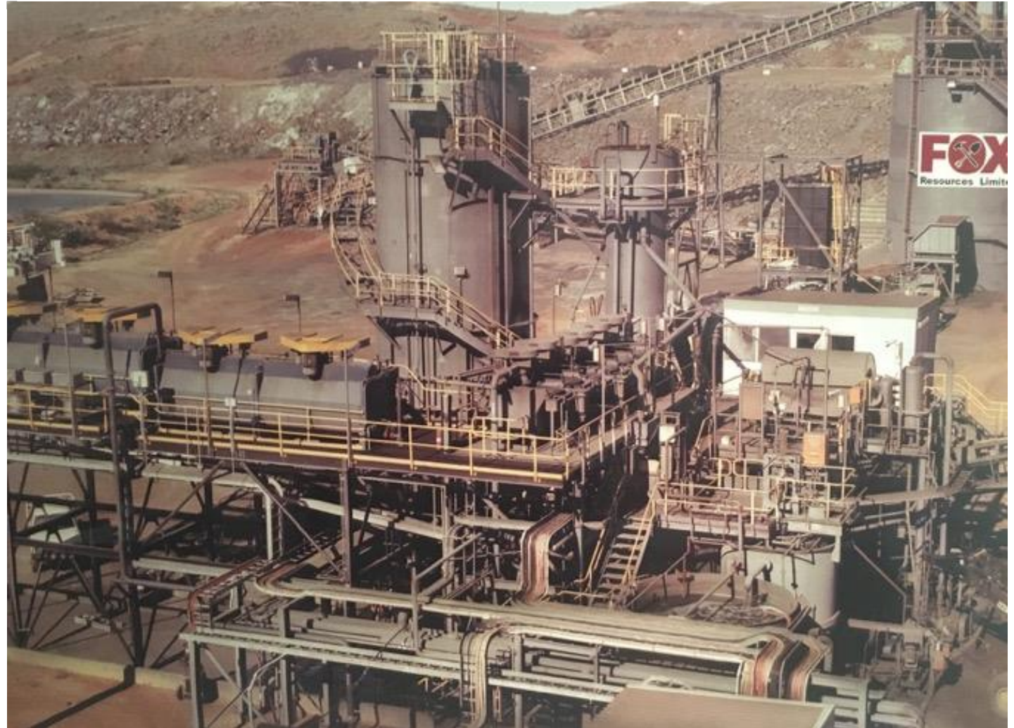
425,000 tpa Radio Hill Treatment Plant – Karratha, WA
