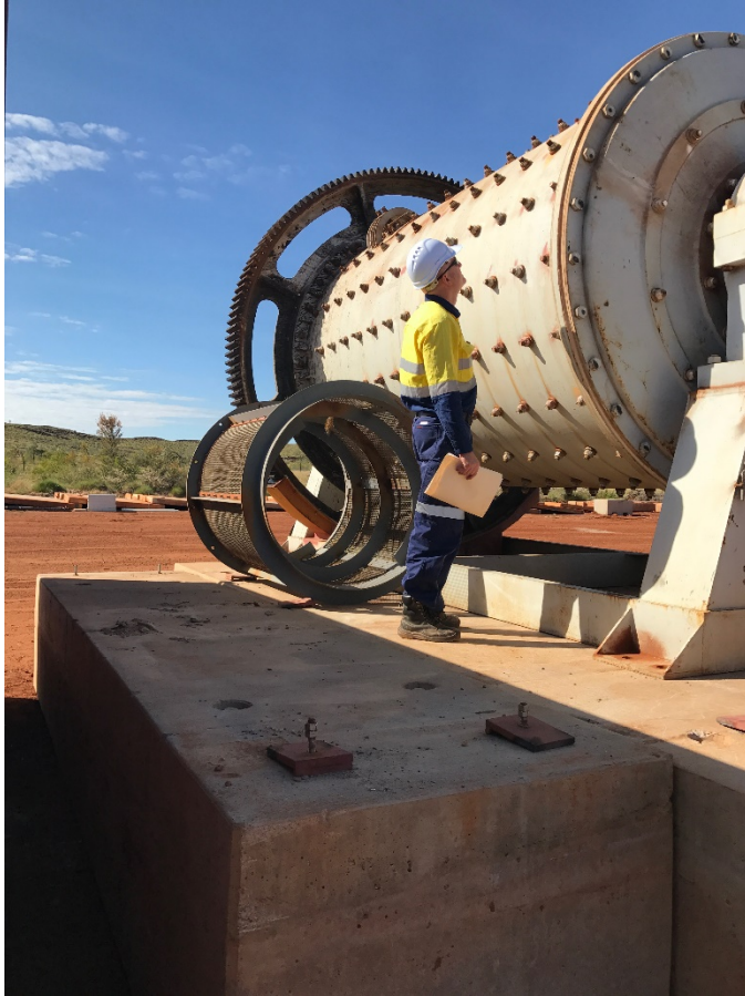
Figure 1: Ball Mill on foundations
