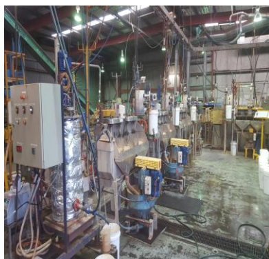
Beneficiation Pilot Plant
