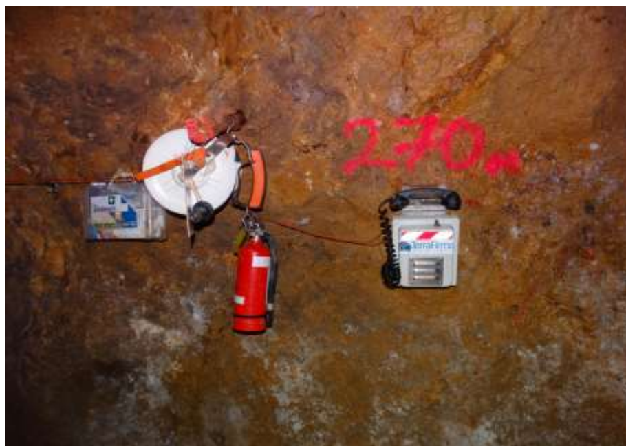
Figure 5 – Communications underground at 270M mark
