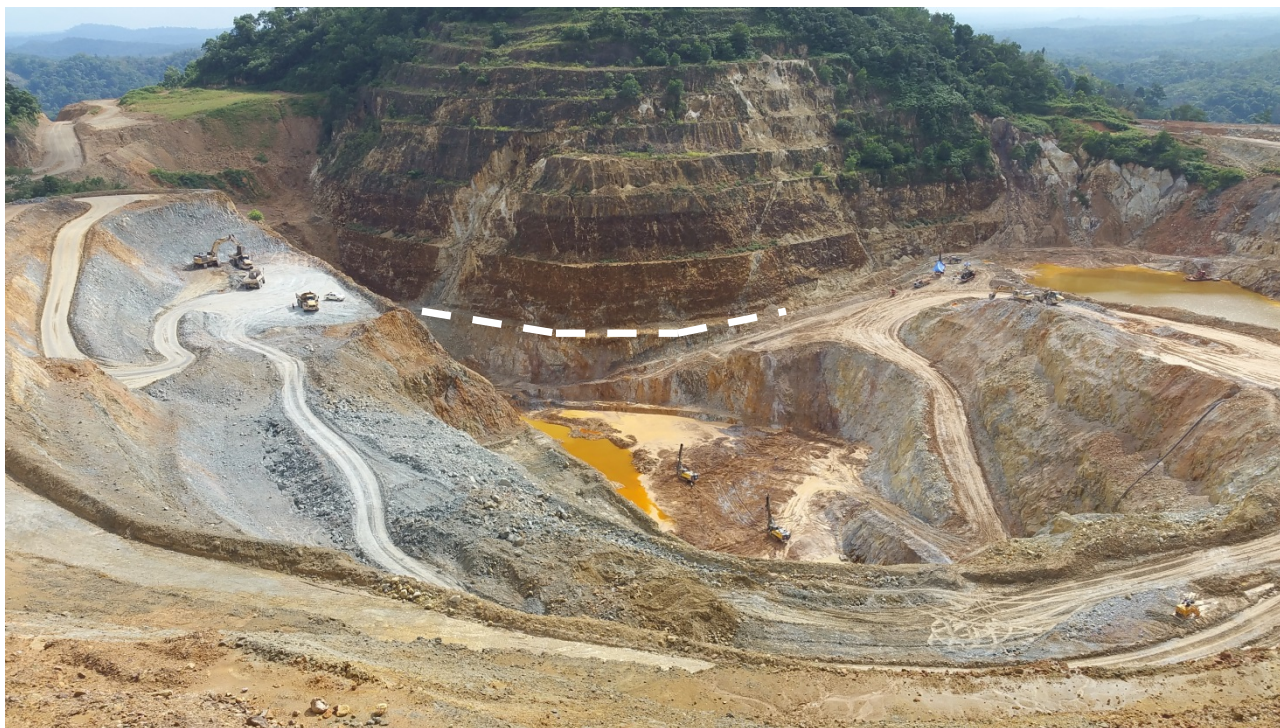
Figure 6. Berenai pit after mud removal. The white dashed line depicts the mud level from March quarterly report photo.
