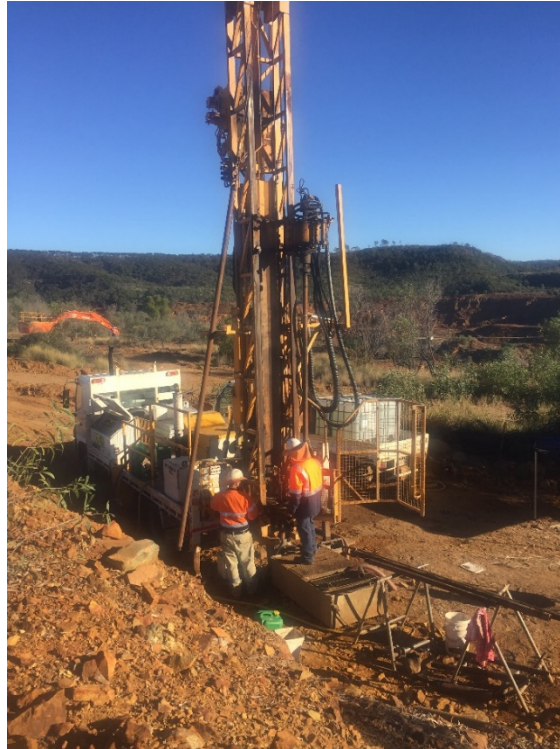
Figure 1 – Geotechnical drilling occurring at the proposed processing plant site at Mount Morgan
