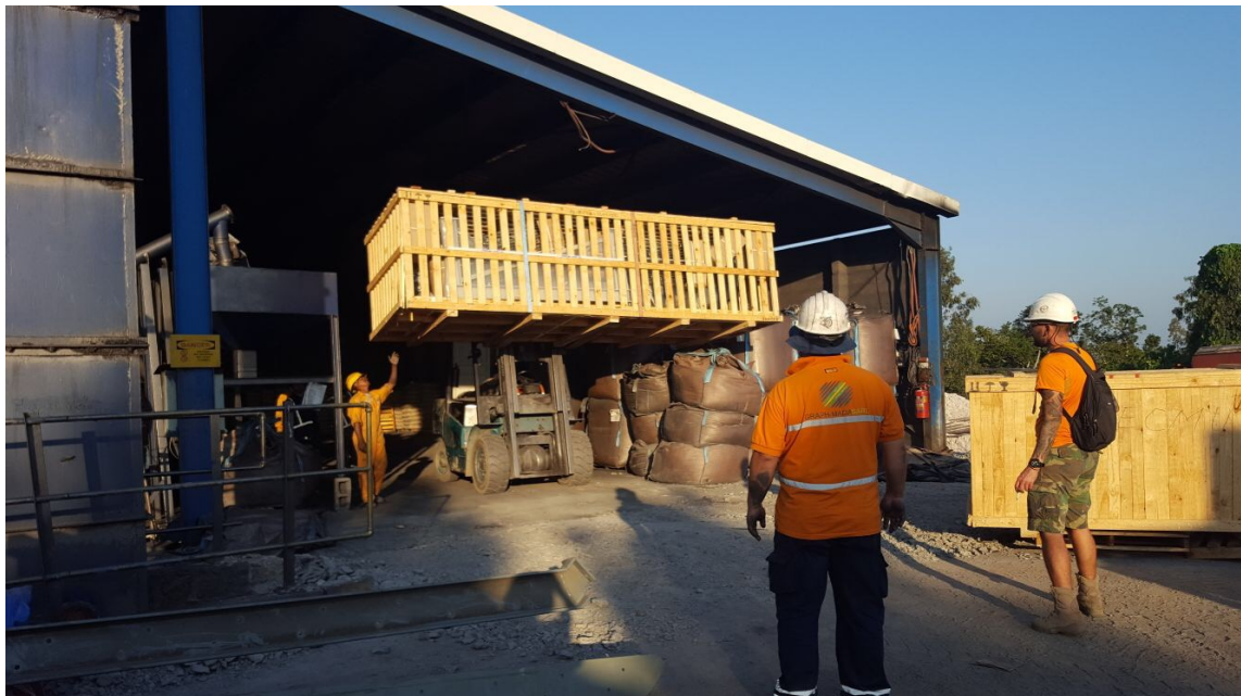
Figure 2: Modular Drying System components being temporarily stored in the Product Storage Facility.
