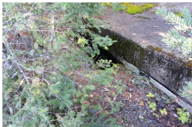
Image 8: Concrete slab over the entrance to the shaft at the Van Chester (Last Chance) Prospect
