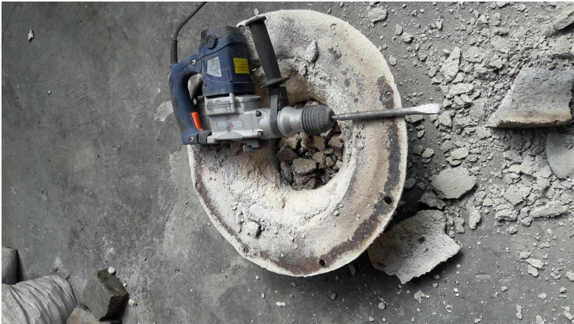
Photo 14. Furnace being relined by removing of the entire pre-existing aluminium cement refractory liner (front cover).
