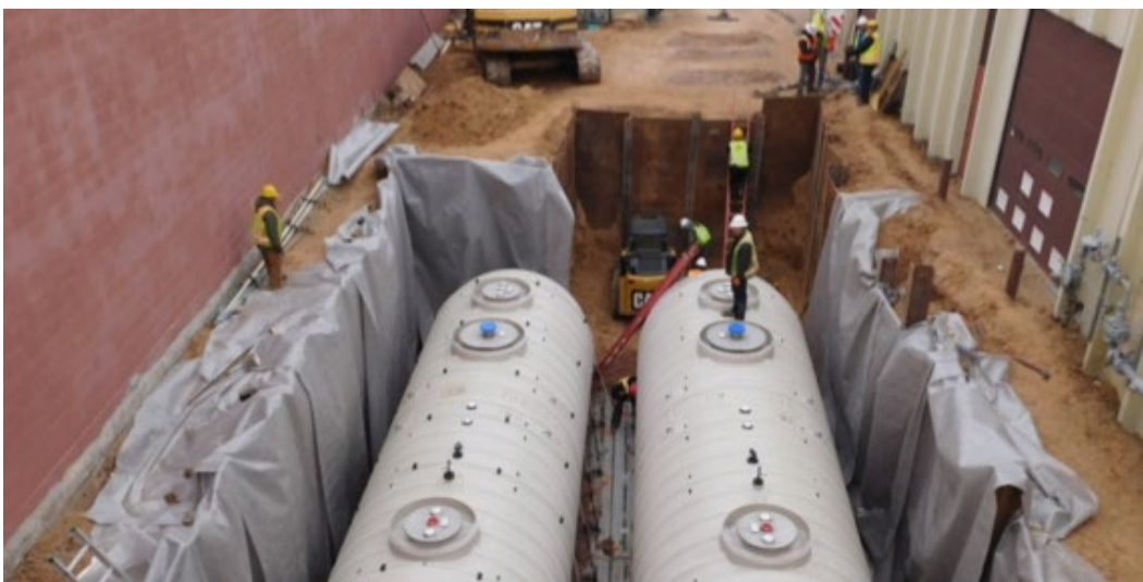
Figure 2. Two 20,000 gallons capacity EdenCrete® underground storage tanks.
