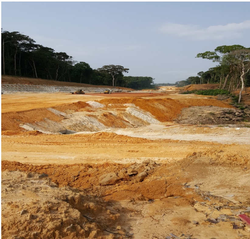
Figure 3: Construction underway of the road and rail corridor immediately east of the Kribi Deep Sea Port
