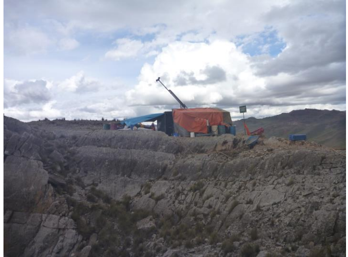
Figure 13: RIGHT The drill rig at RDDH-021. The hole is testing HV-011, a NW-SE trending vein believed to splay west from the Callancocha Structure. This hole is the first hole drilled at Humaspunco West.
