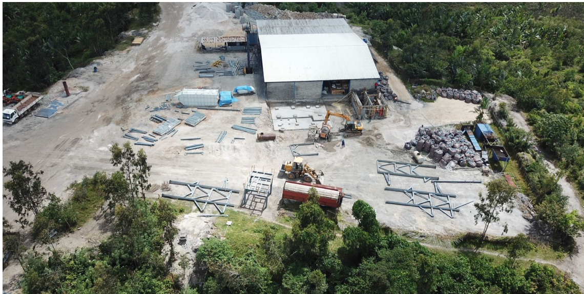
Figure 1: The commencement of MDS installation; laying out of frames, completion of structural footing, and control room construction nearing completion.
